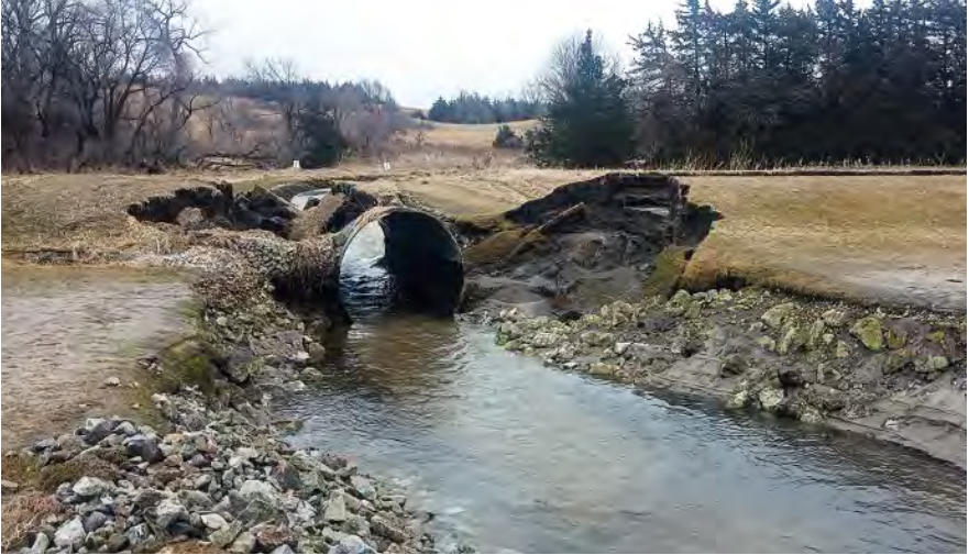
A culvert on the East Branch of Verdigre Creek at the Grove Trout Rearing Station washed out March 14. Quick repairs were required so hatchery staff could access trout in the raceways and ponds.
