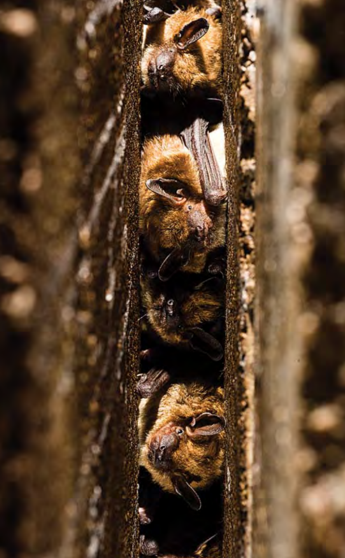
Hundreds of big brown bats roost in gaps between concrete sections of an abandoned building at Camp Ashland, a Nebraska National Guard facility near Ashland.
