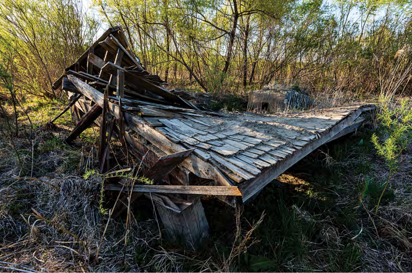
Following the flood of 2019, the shelter's roof collapsed and the fireplace toppled. ERIC FOWLER, NEBRASKALAND
