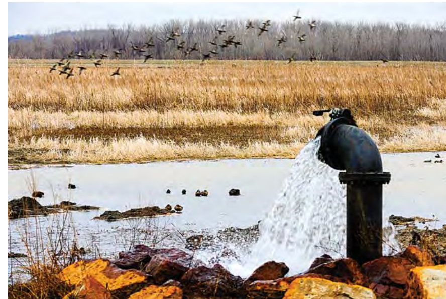
Teal circle a wetland as well water, pumped to provide wetland habitat during the spring migration, pours from a pipeline riser.
